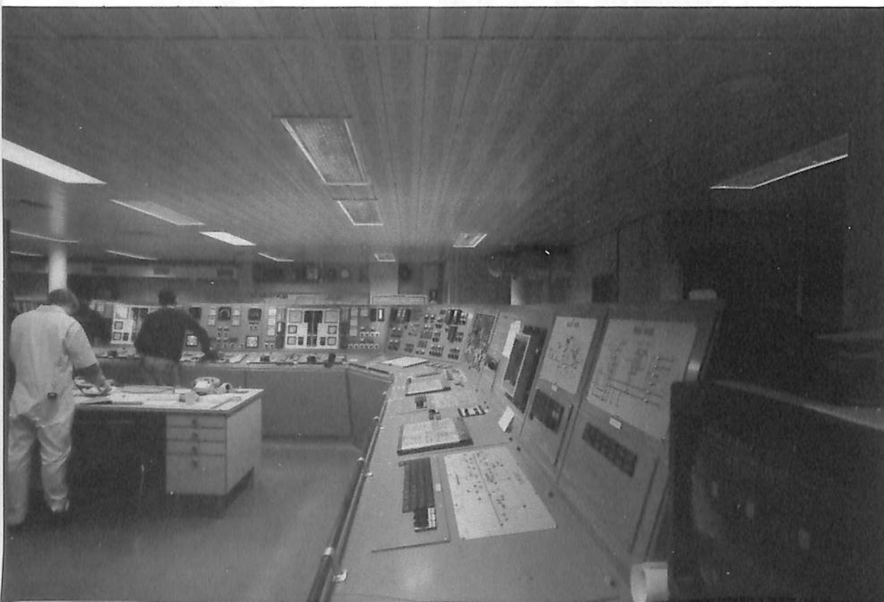
▼ Engine Control room
