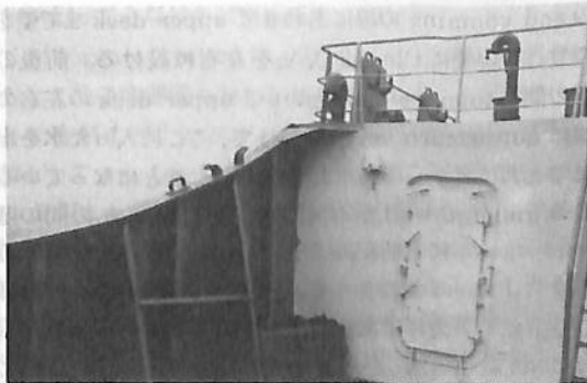
Fig. 3 Class 1 Closing appliance (watertight door)
