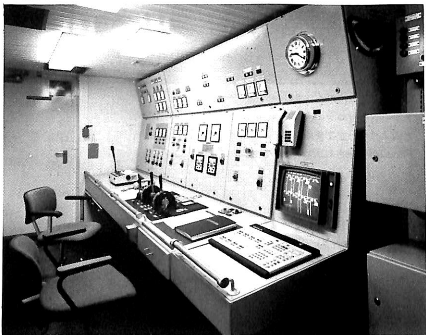
Engine control room
