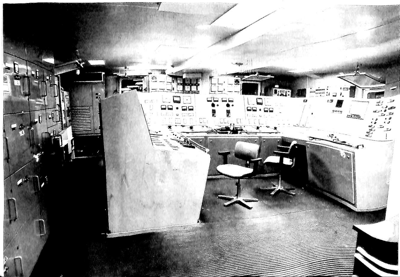
Engine control room
