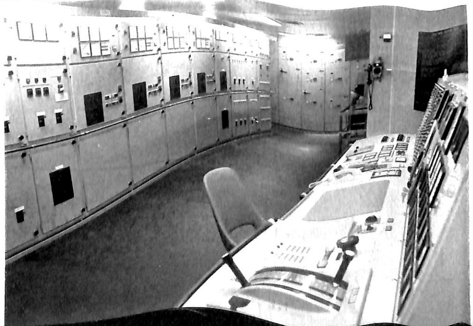
Engine control room
