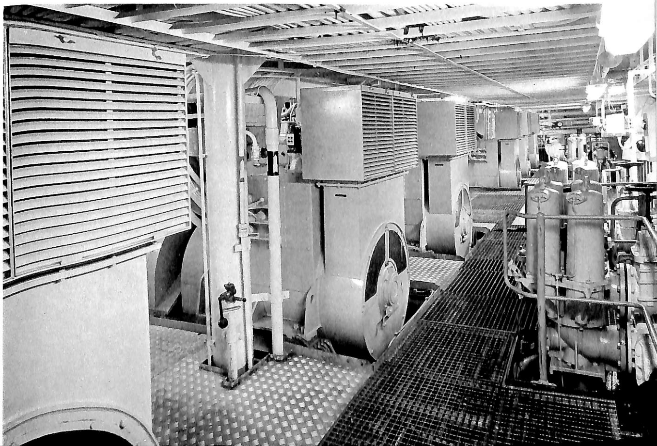
Auxiliary engine room
