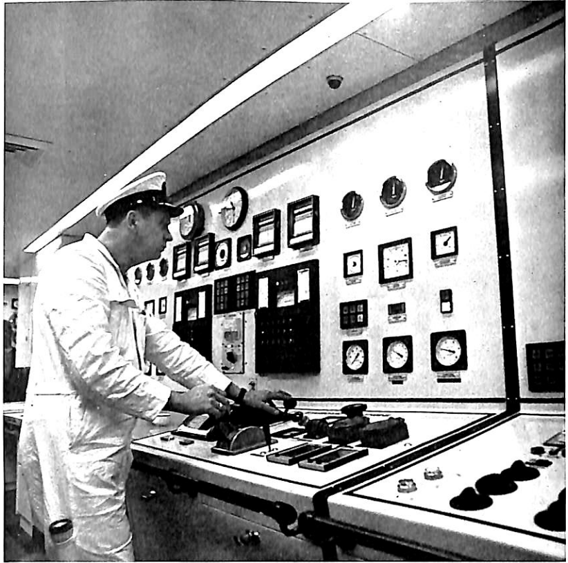
Engine room control console
