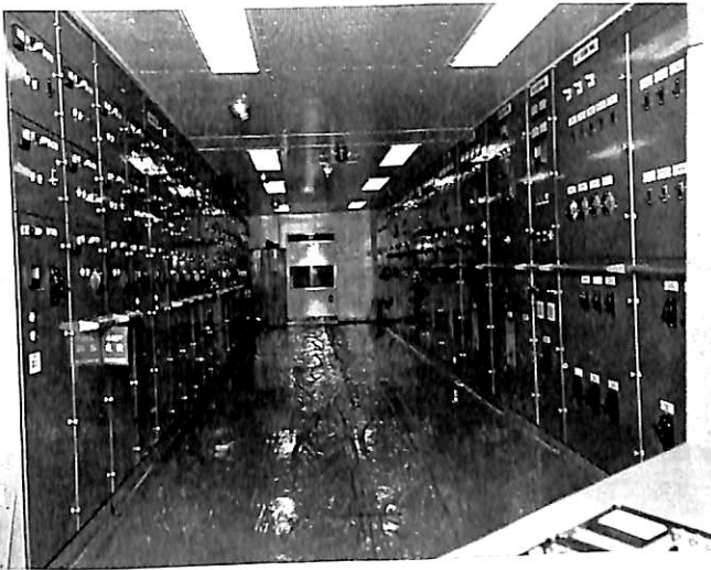
Engine Control Room (main switch board)
